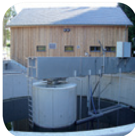
Station d'épuration, Mamach - Luxembourg Wastewater treatment plant
