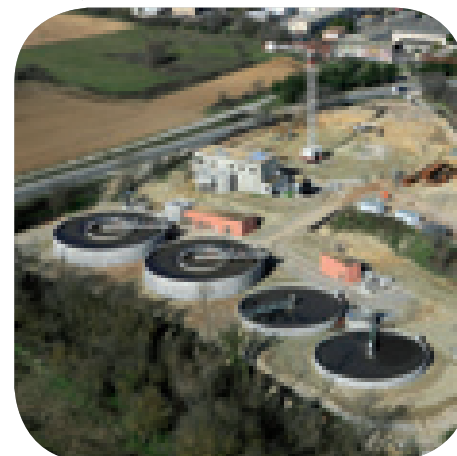
Station d'épuration, Fabrègues (34) Arch. : Agence Coste Architecture Wastewater treatment plant
