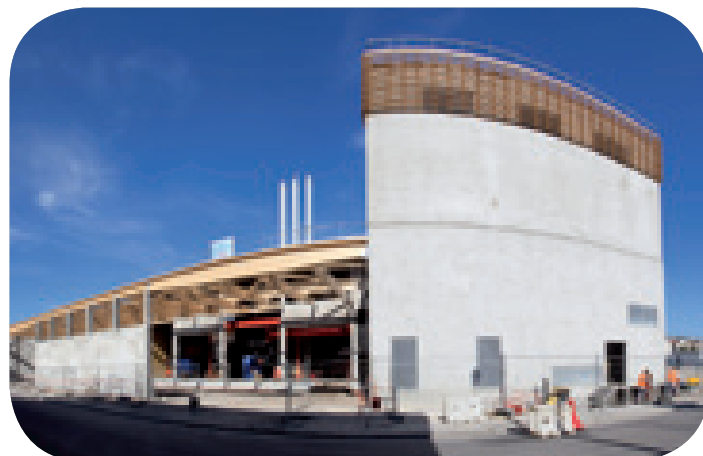
Chaufferie biomasse, Nancy (54) Arch.: B.M.T Biomass boilers fuelled
