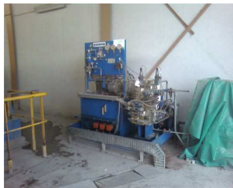
Figure 9:installation de freinage.
